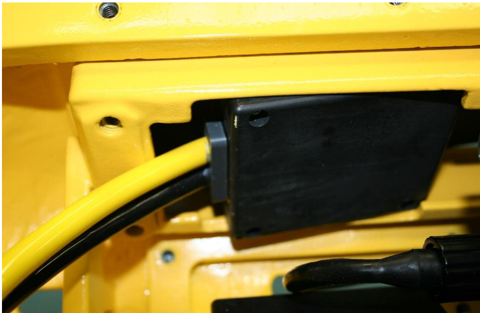
Figure 2-12: Cable in Keyway
