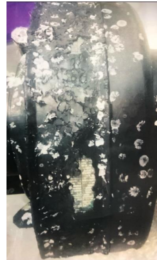
Cleaning of system with a power washer, causing exposure of the ceramics.
